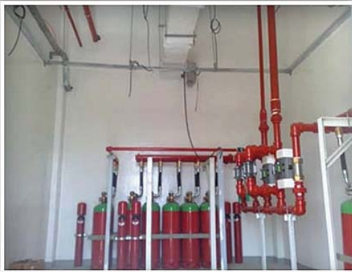
FM200 Firefighting & alarm system Client : Tanmia for oil field services
