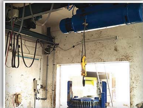
supply and install of electrical mobile lifting 5 Ton crane at pump Station No.2 Hodiedah City Client : ICRC
