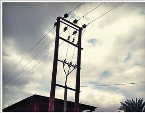
Supply, Install and repair 11kv TL. for Bajil water system Client : ICRC
