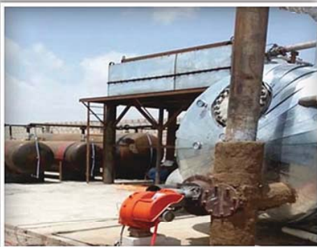
Oil recycling plant Client : AL-kawon Company
